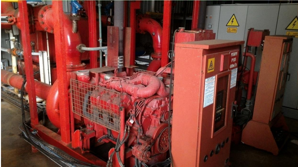
Figure 55 : Pomperie incendie diesel
